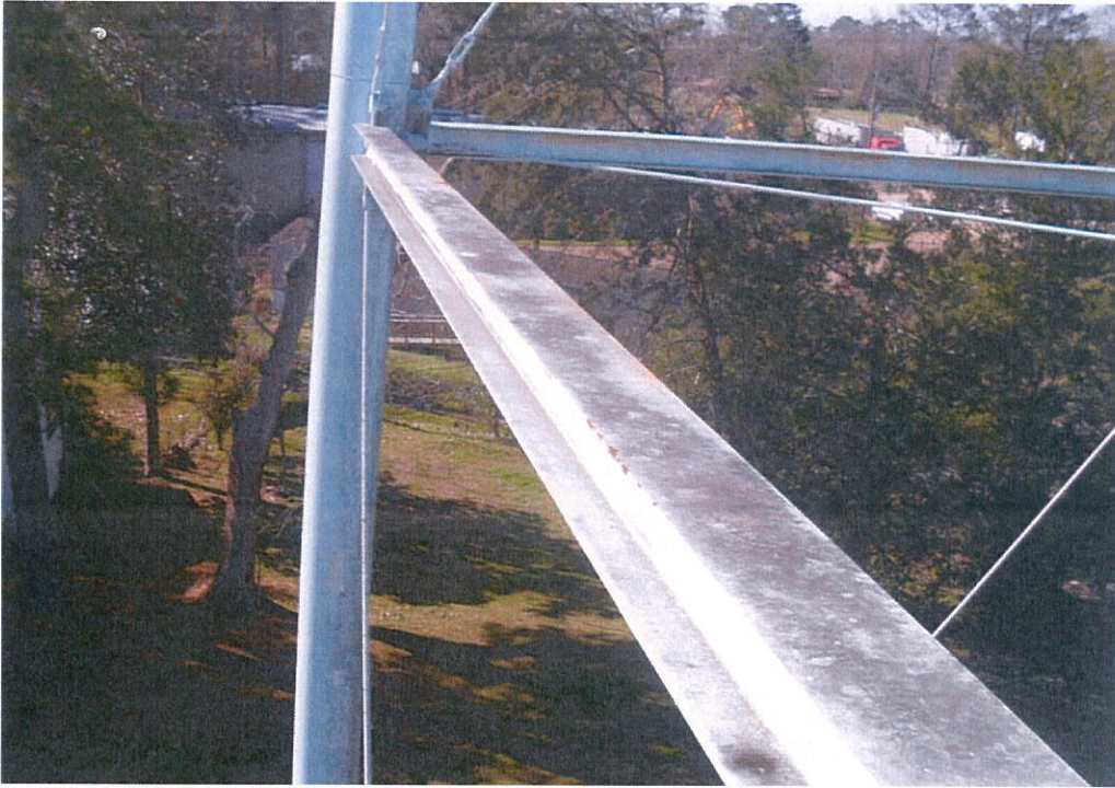
Figure 11. Heavy mold and mildew on first level struts
