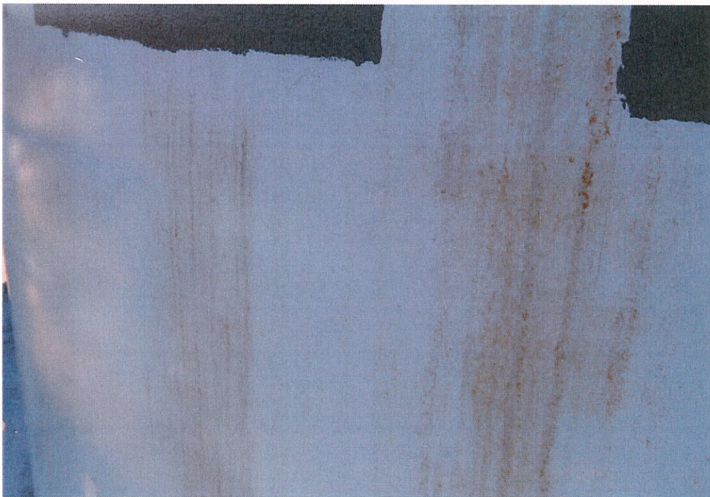
Figure 22. Coating failure on shell wall
