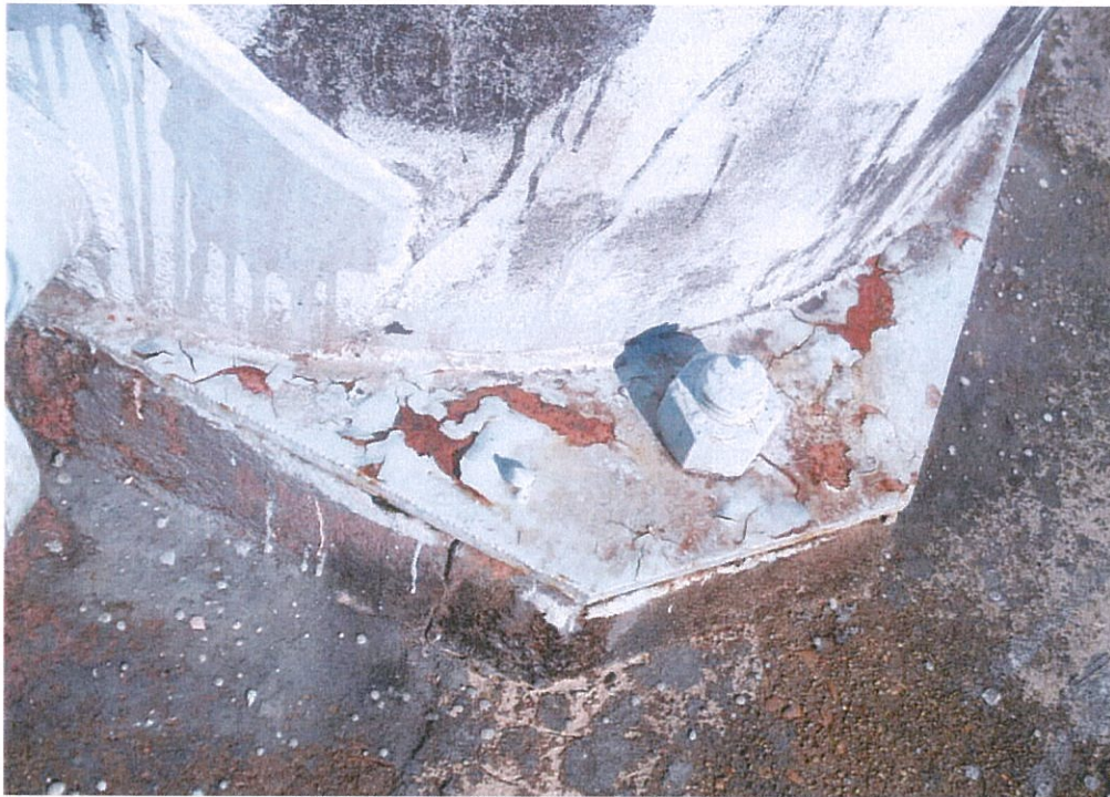
Figure 7. Coating failure on riser foundation
