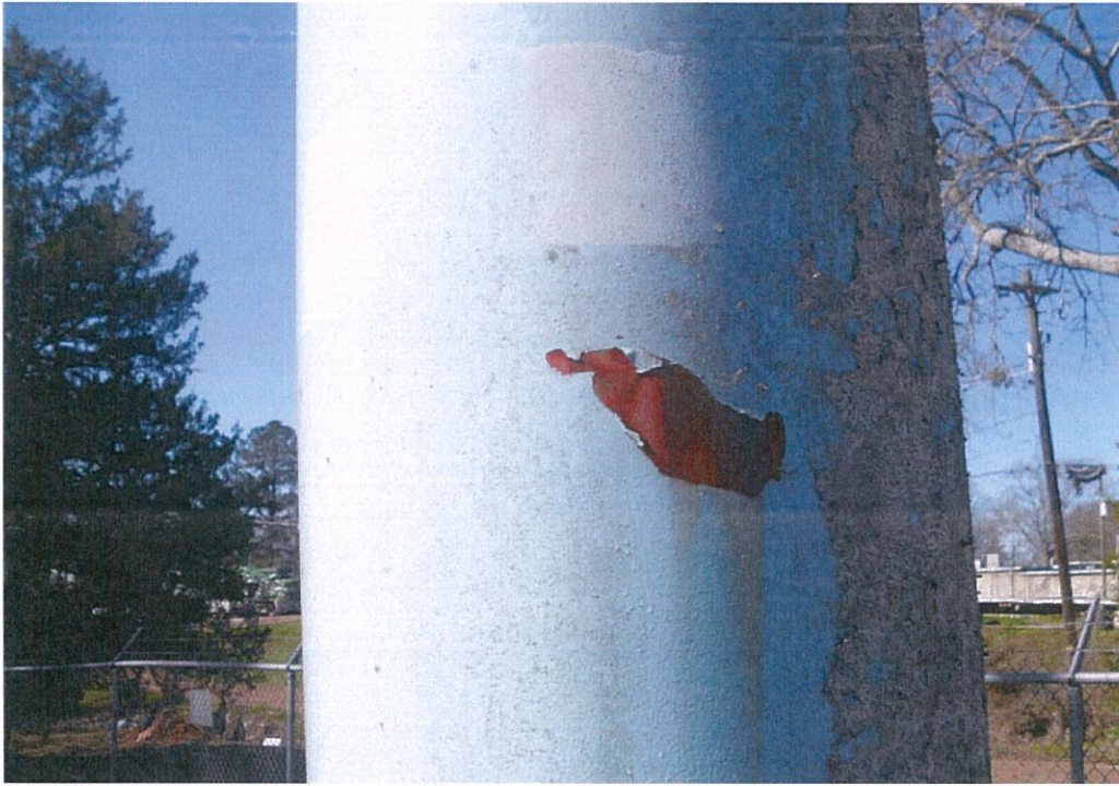
Figure 5. Coating failure on tank column
