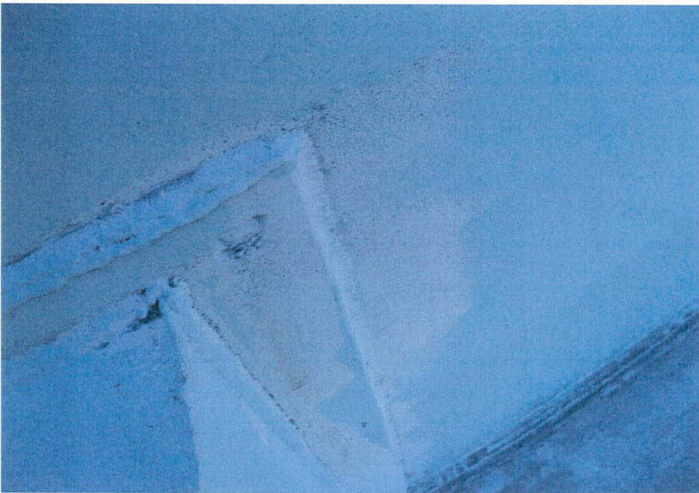
Figure 26. Uncoated area on tank column flange above balcony
