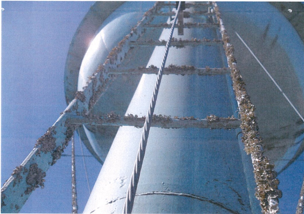
Figure 13. Heavy lichen growth on tower ladder
