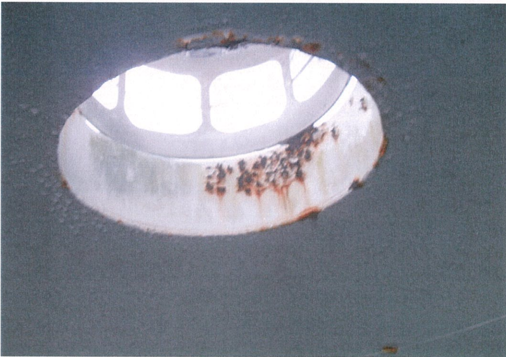
Figure 38. Coating failure on tank roof vent
