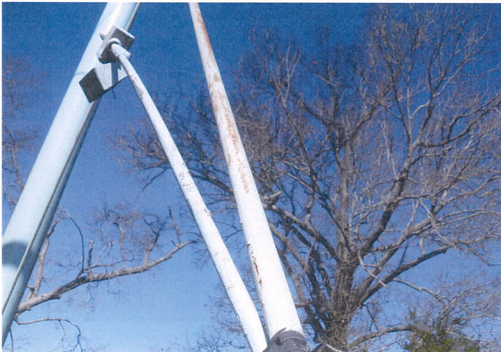
Figure 10. Coating failure on wind rod and broken electrical conduit
