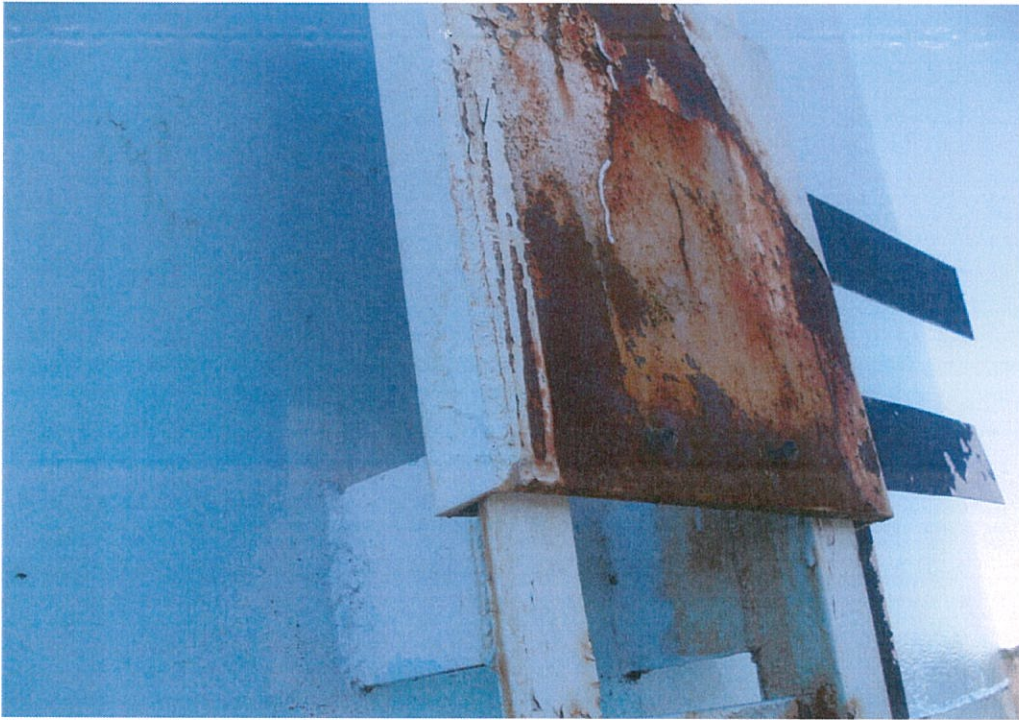
Figure 25. Coating failure on tank level indicator
