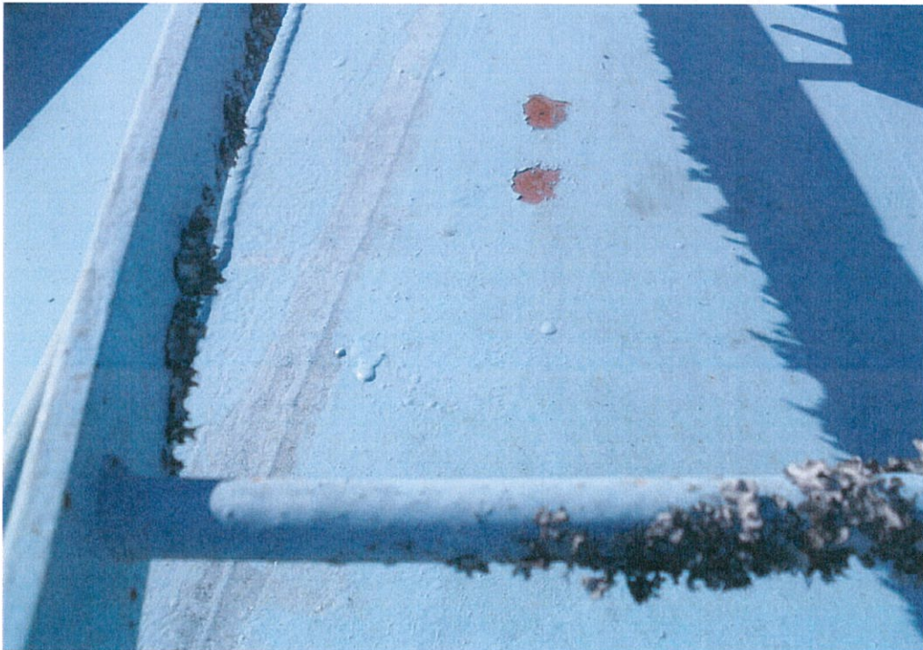
Figure 27. Area missed during last coating and two localized areas of coating failure on roof of tank.
