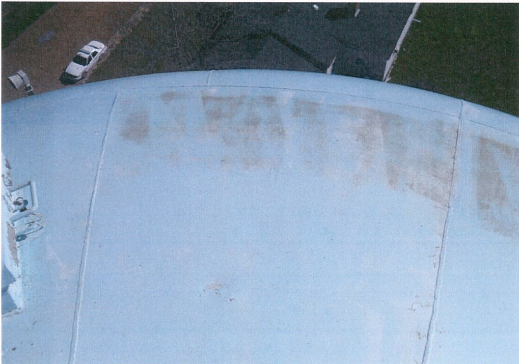
Figure 30. Coating failure on roof of tank
