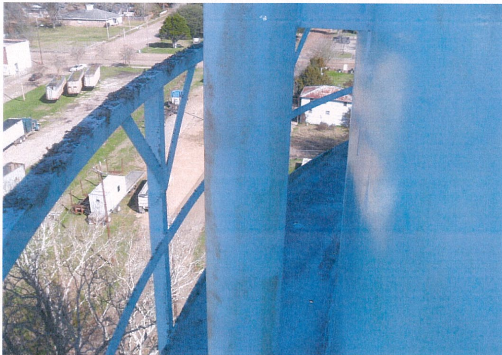
Figure 23. Coating failure on overflow
