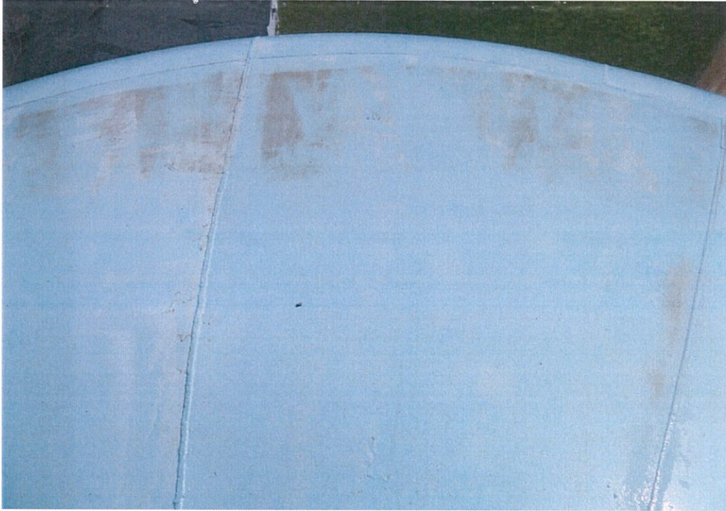
Figure 29. Coating failure on tank roof
