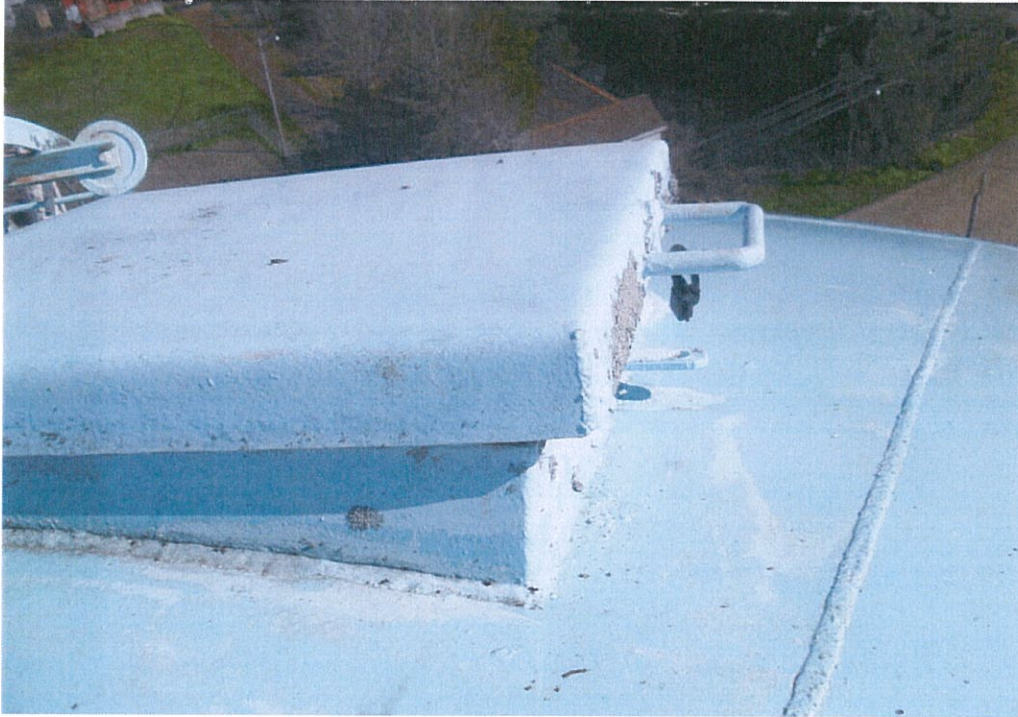
Figure 31. Unlocked hatch. Door is warped, lock wouldn't reach.
