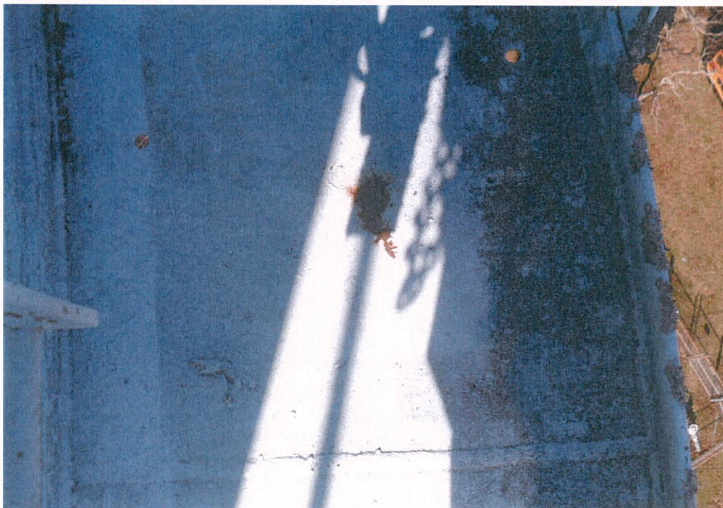
Figure 24. Coating failure on balcony floor
