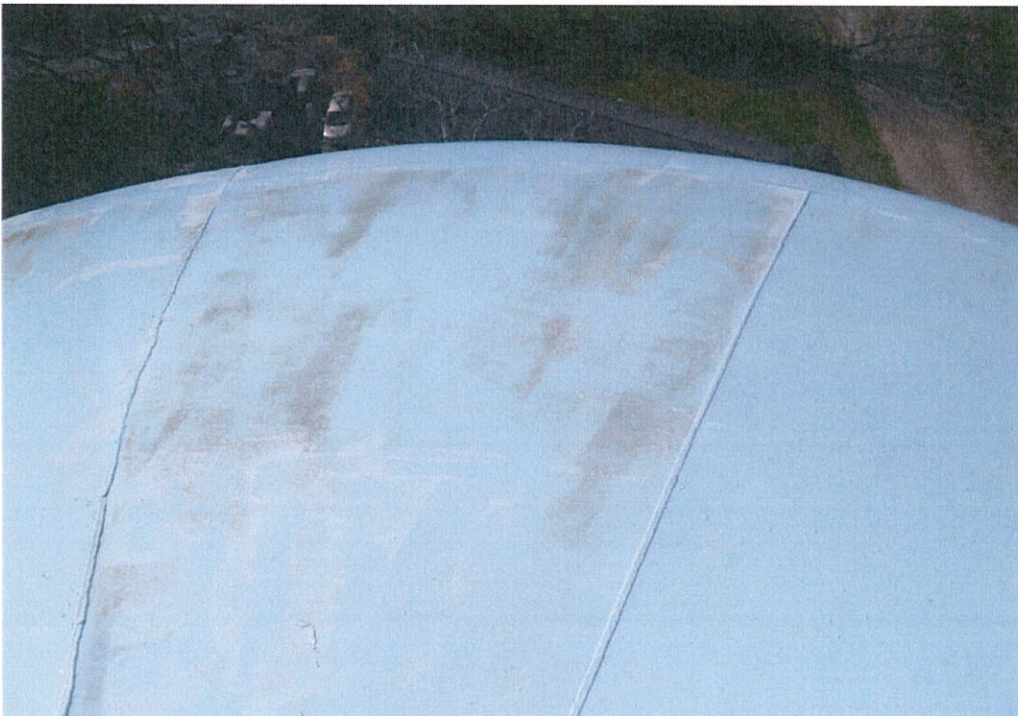
Figure 28. Coating failure on roof of tank
