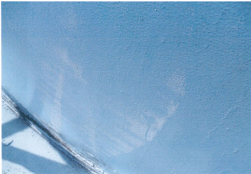
Figure 16. Area missed during last coating on tank shell wall
