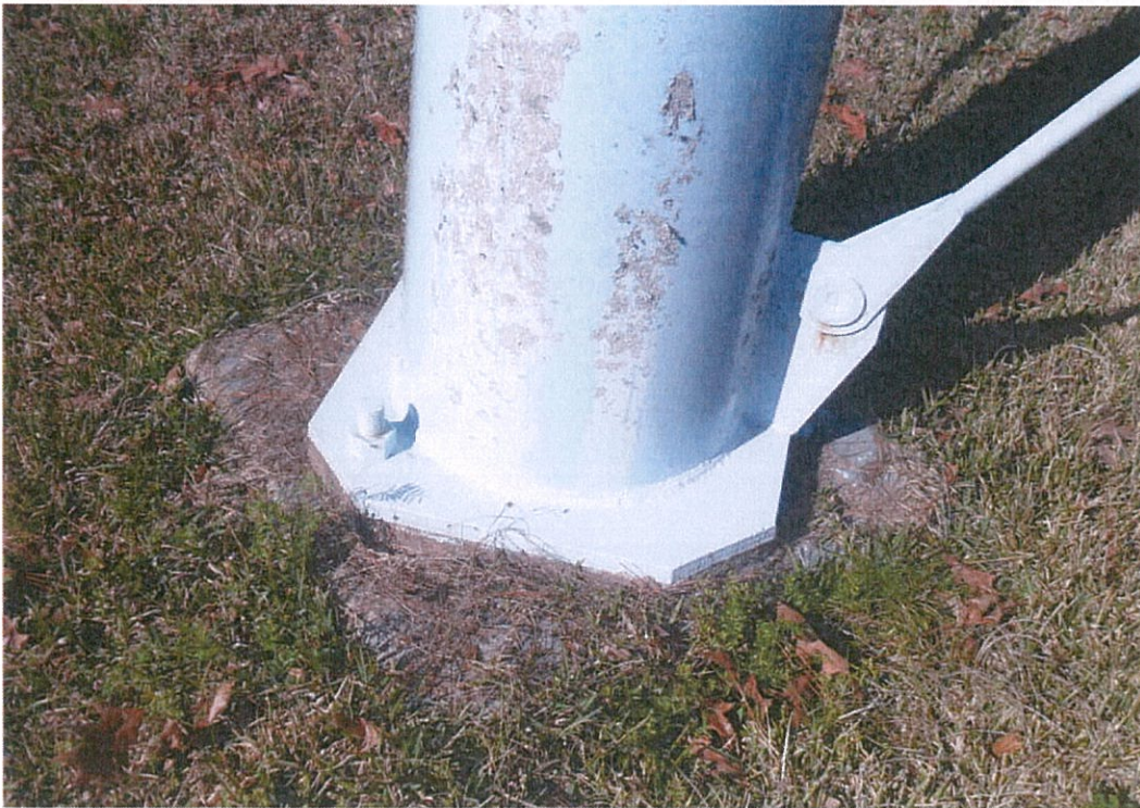
Figure 2. Condition of tank support foundation
