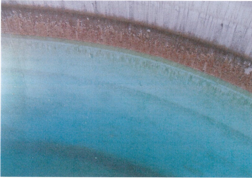
Figure 37. Heavy sediment on interior wall
