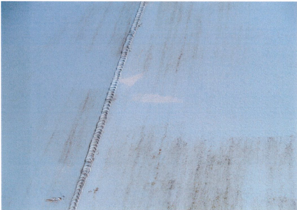
Figure 20. Coating failure on shell wall
