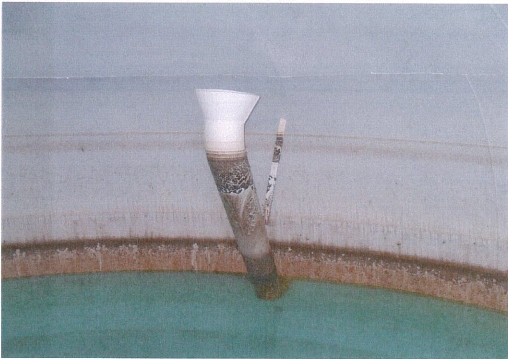
Figure 32. Heavy sediment on interior wall and overflow
