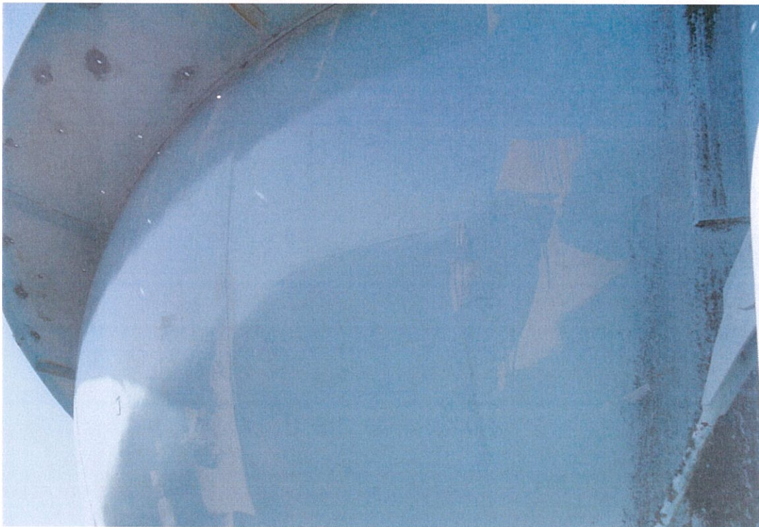
Figure 14. Areas that were missed during the last coating
