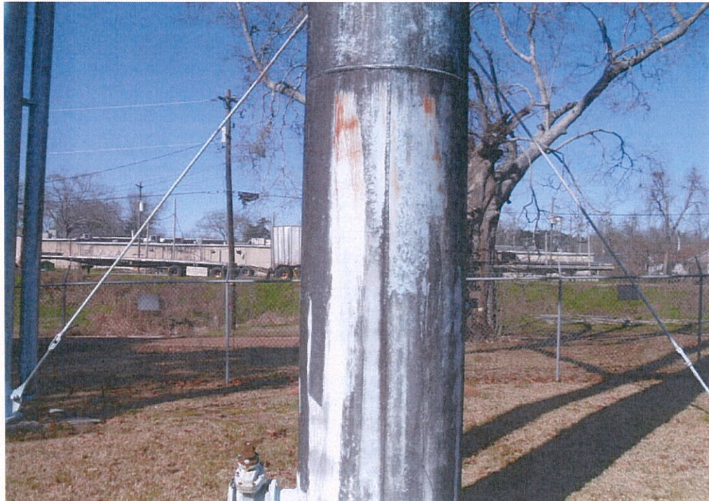
Figure 6. Coating failure on riser
