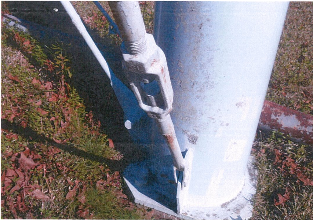
Figure 9. Coating failure on wind rods
