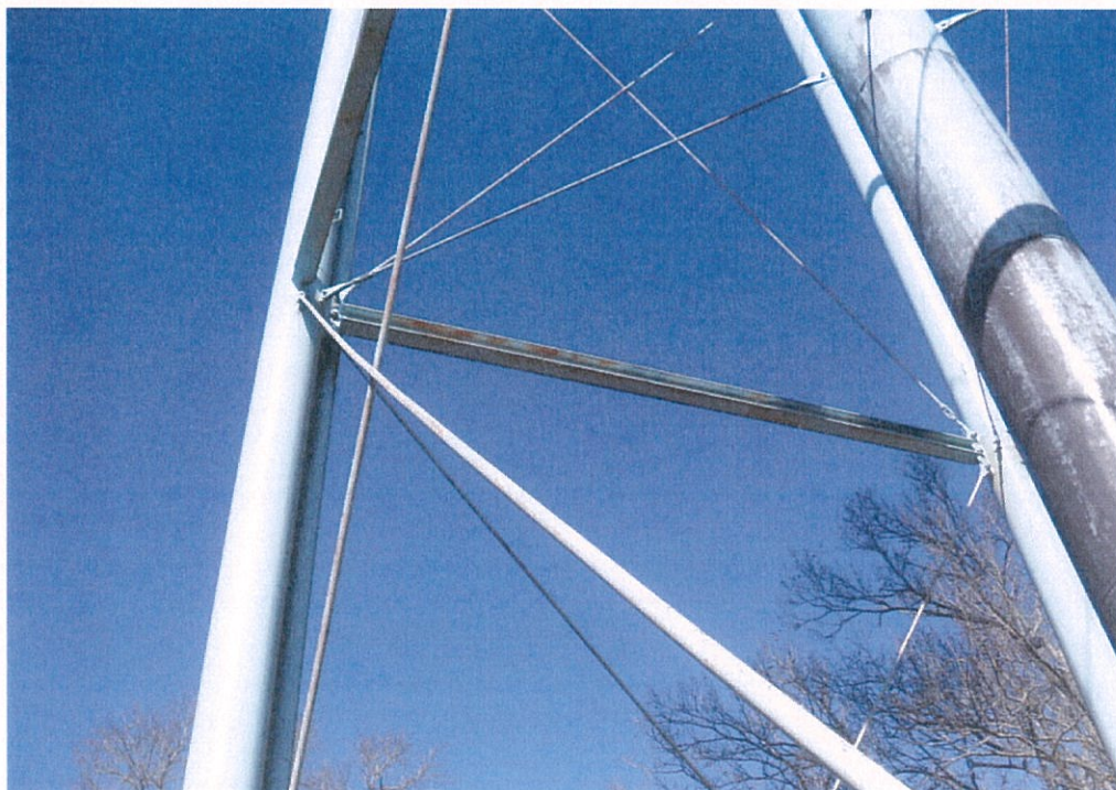
Figure 4. Coating failure on struts and heavy mildew on riser
