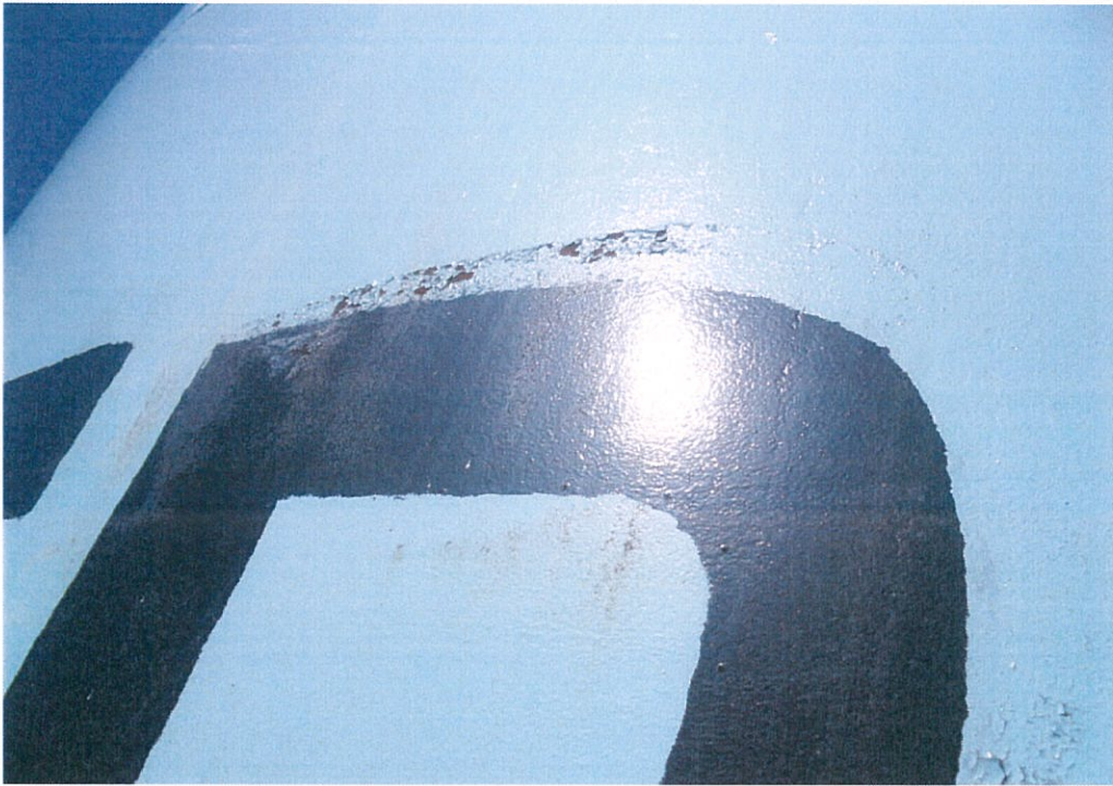
Figure 19. Small area of coating failure on shell wall
