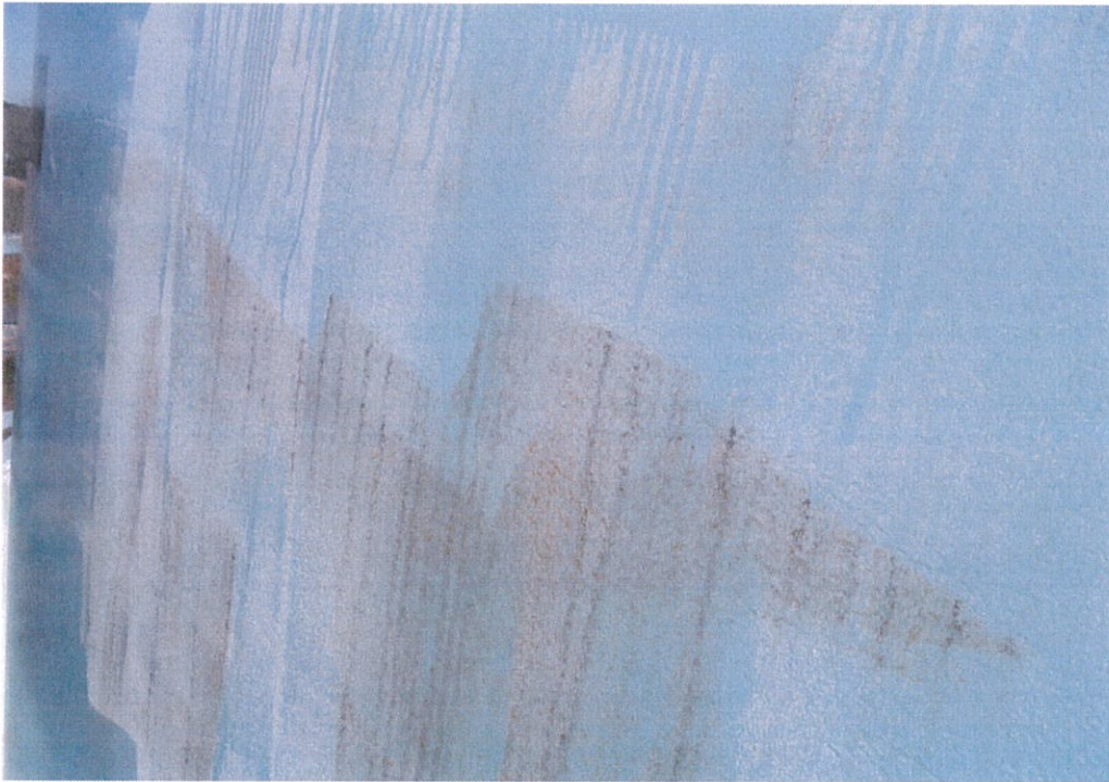
Figure 21. Coating failure on shell wall
