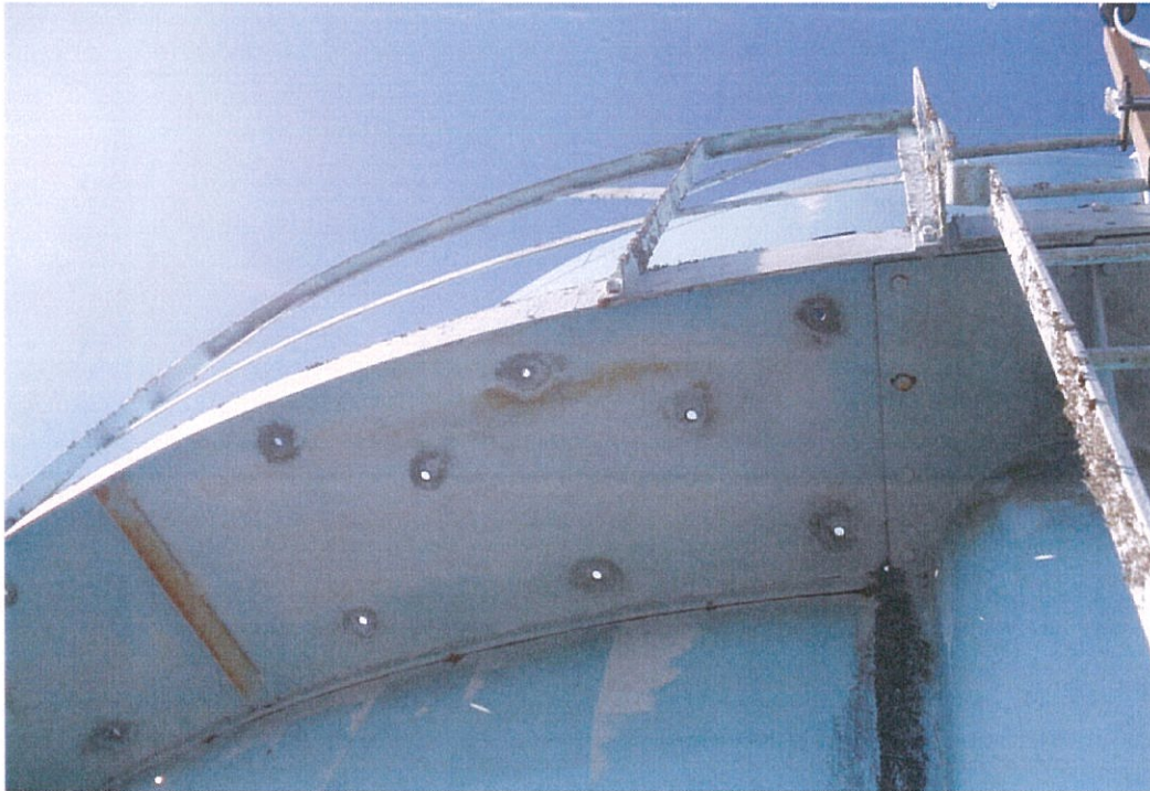
Figure 15. Coating failure under balcony floor
