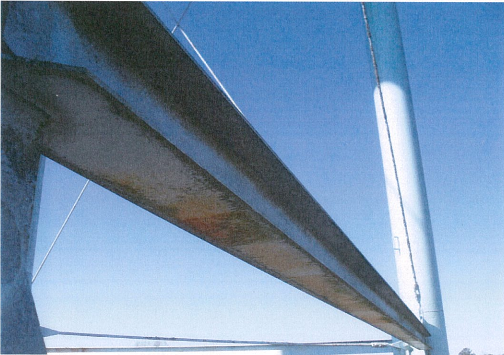
Figure 12. Coating failure on first level struts
